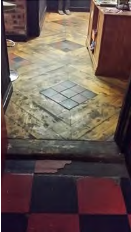
Step requires temporary or permanent ramp, bar area has a confusing surface & bar furniture. The accessible toilet is on the right in this image.
